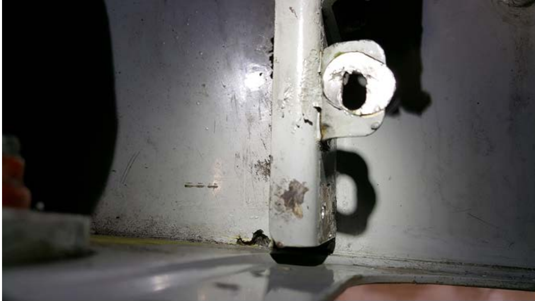
Figure 1 – Corrosion as seen before repair.
