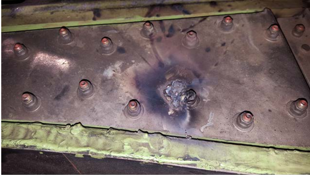
Fig 3: RJ900 - Fastener damaged by arcing
