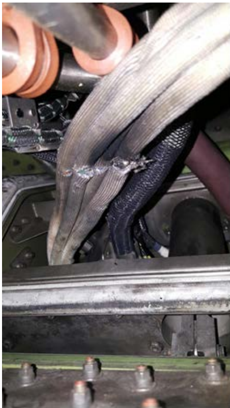
Fig 4: RJ700 – Damage to wires
