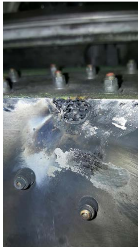
Fig 5: RJ700 – Damage to fastener and panel
