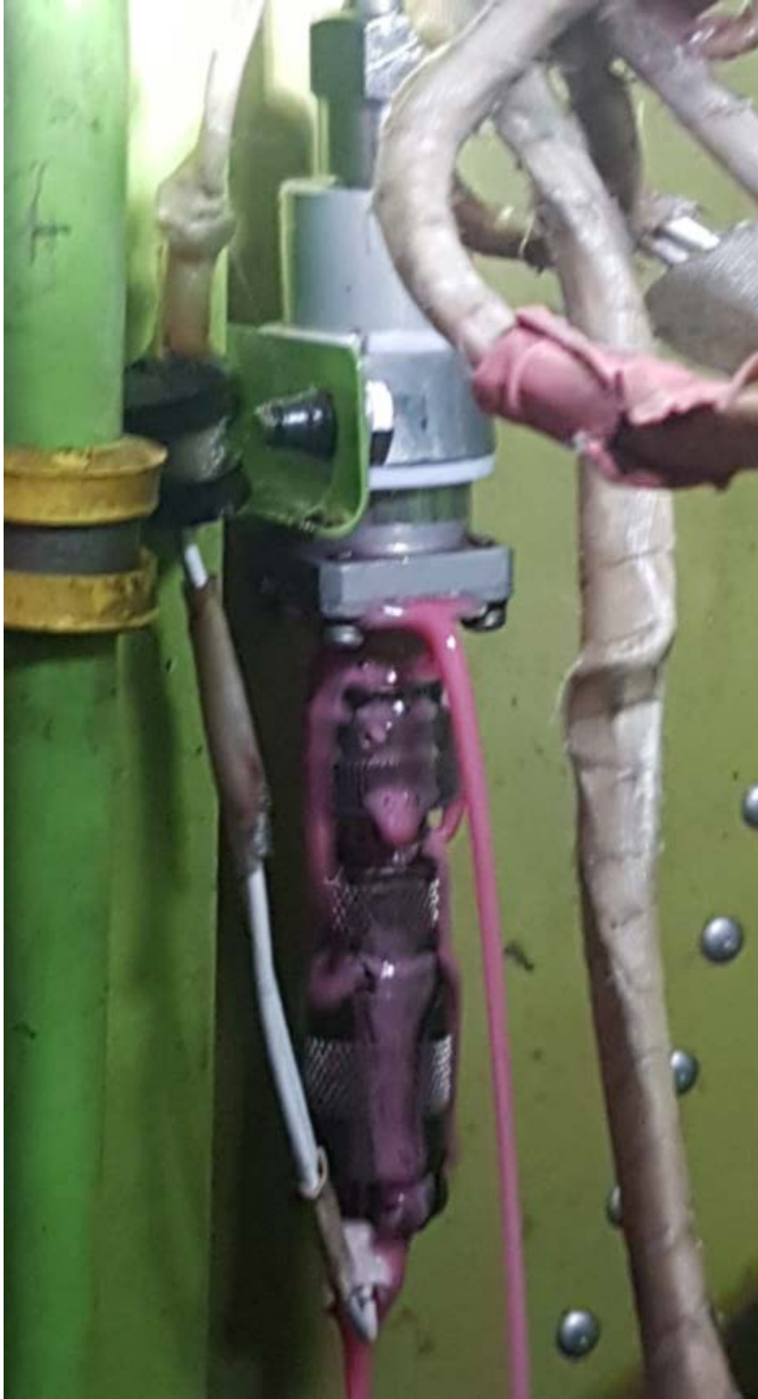
Pic#1 – Low pressure switch S9 leak
