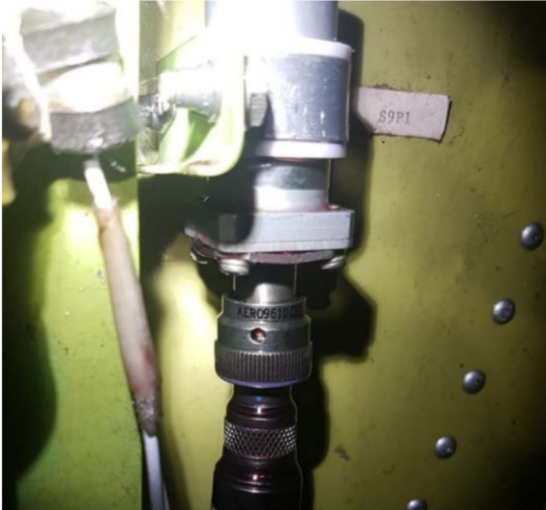
Pic# 2 - Bulge in connector body and subsequent protruding O-ring
